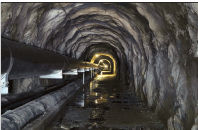
Water tunnel of 600 km, under construction in Yunnan, is part of a pilot project to test technical capabilities to construct the Tibet-Xinjiang tunnel. Photo: Wikimedia commons
